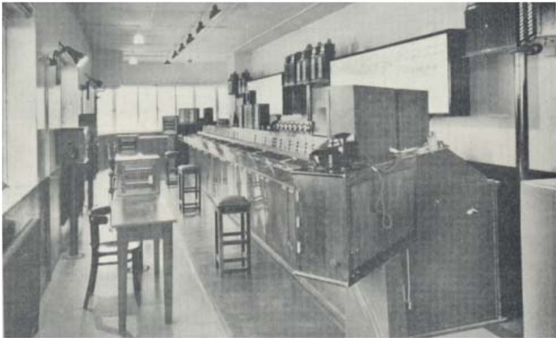
The 131-lever power frame, with illuminated diagrams and train describers, at Gloucester Road Junction Signalbox
